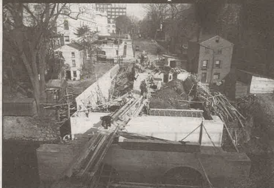
This photo shows construction workers building the Prospect Street Bridge over the Park River in the early part of the 20th century. The view is looking north; City Hall can be seen at upper left. Prospect Street is one of Hartford's oldest streets. Hartford founder Thomas Hooker lived on the east side of the street, which was then just a pathway, on the banks of the Park River. In 1687, when Joseph Wadsworth grabbed the royal charter at a meeting held near where the Travelers Tower stands today, and hid it in the Charter Oak Tree, he probably ran down Prospect Street. A monument to the Charter Oak stands at the corner of Prospect Street and Charter Oak Avenue. (Photo courtesy of the Hartford History Center at the Hartford Public Library)
